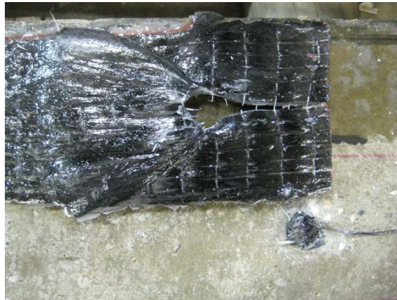
Figure 3.20 Detail of anchor fracture
