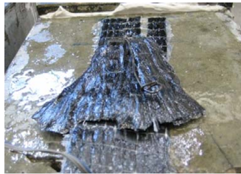
c) Debonding of CFRP anchor
